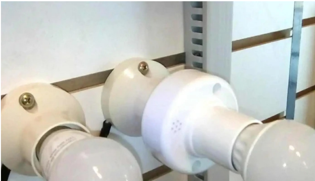
Electro interior interior
